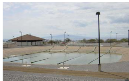
Lined Earthen Aeration Basins
