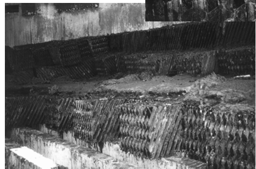
Photo 4: Collapsed Media Layer
